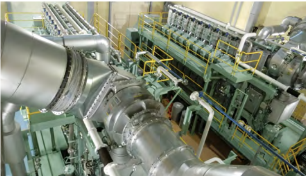
Gas engine power generation facilities
