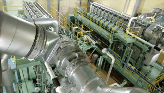
Gas engine power generation facilities
