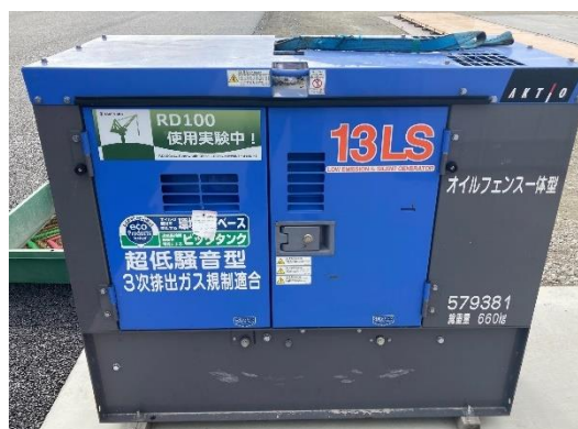
A power generator operated with RD
