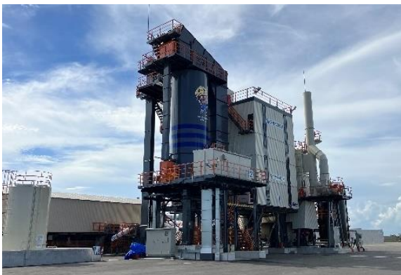
Omuta asphalt plant
