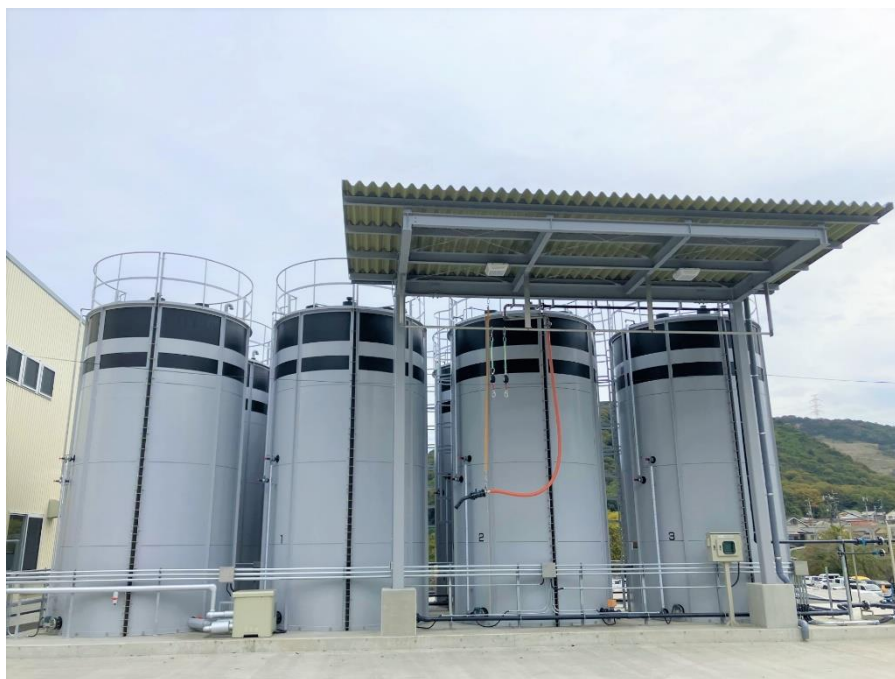
AdBlue storage tanks installed in the new manufacturing plant
