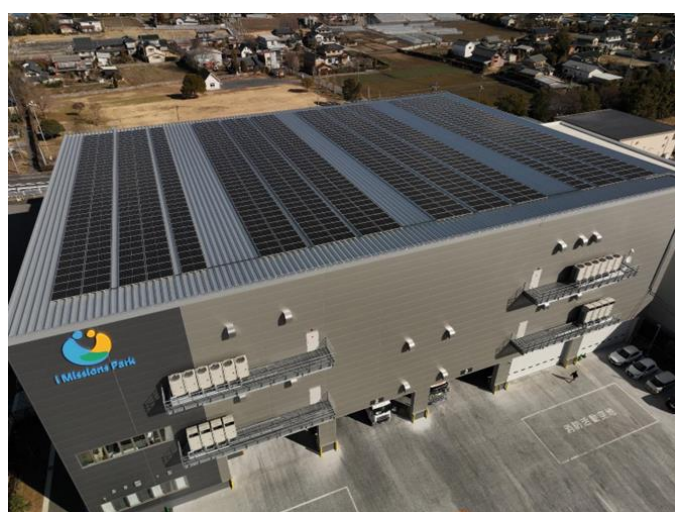
① Solar power plant of i Missions Park Kazo
