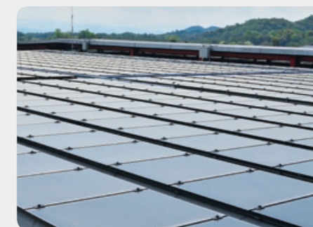
A photovoltaic power generation system installed on the roof of a cattle shed (Masuda City, Shimane Prefecture)
