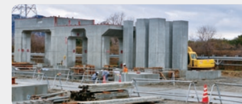
Coal thermal power generation plant currently under construction (Hofu City, Yamaguchi Prefecture)
