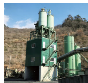
Fly ash reuse facility
