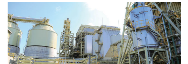
Thermal power plant, Sendai Power Station Co., Ltd.
