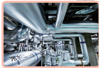
District heat supply facility run by Tokyo Toshi Service Co., Ltd.
