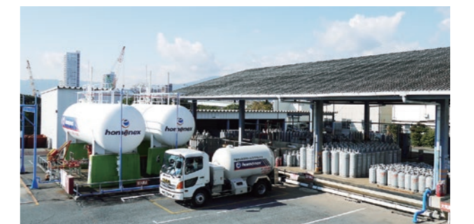
An LP gas filling station, which serves as a storage and supply center
