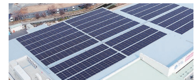
Self-consumption solar power generation facility provided by our Group
